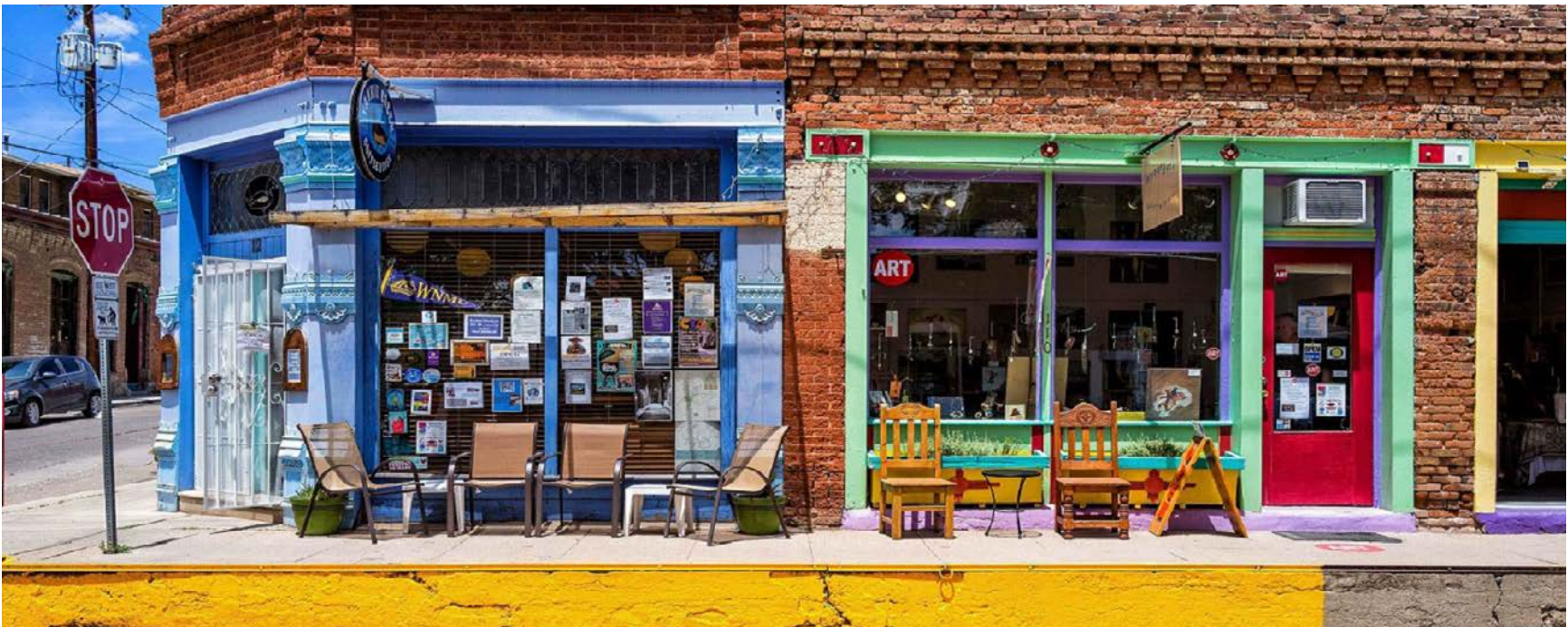
Window frame material different from building material in Silver City, NM
